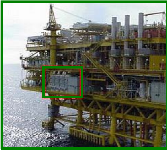
A CO 2 -membrane stripping unit (high-lighted) is attached to an offshore platform operated by Unocal in the Gulf of Thailand. The unit shown here is handling 1.8 mt CO 2 /yr.
